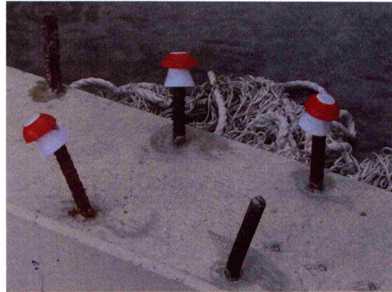
Photograph 2: final state of the protections after the impact.
