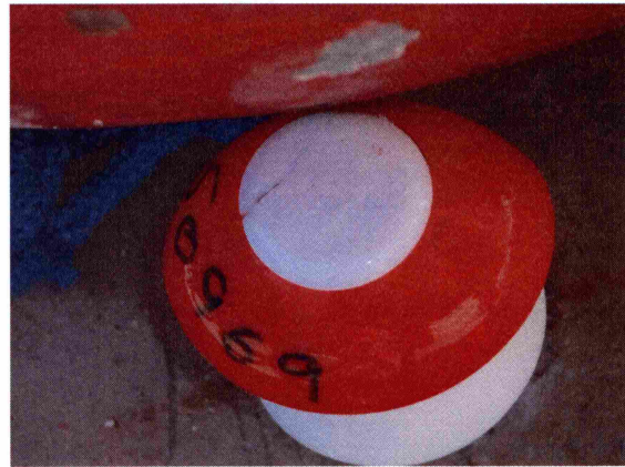
Photograph 8: Detail of the protection after the impact.
