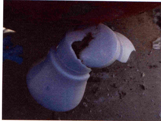
Photograph 10: Detail of the state of one of the protections which has suffered the impact.
